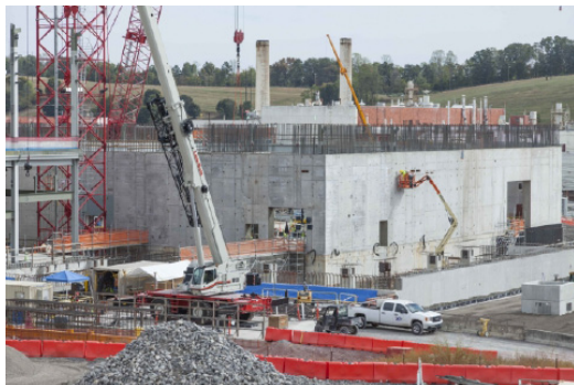
Latest US Bomb Plant, the UPF, under construction, at the Y-12 Nuclear Weapons Complex, Oak Ridge, TN
